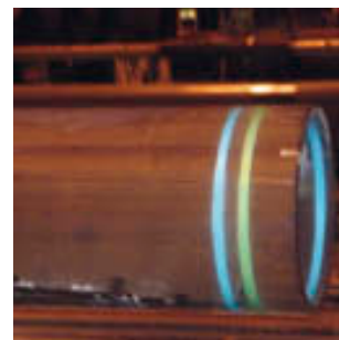
Colored ring marking on steel pipes
